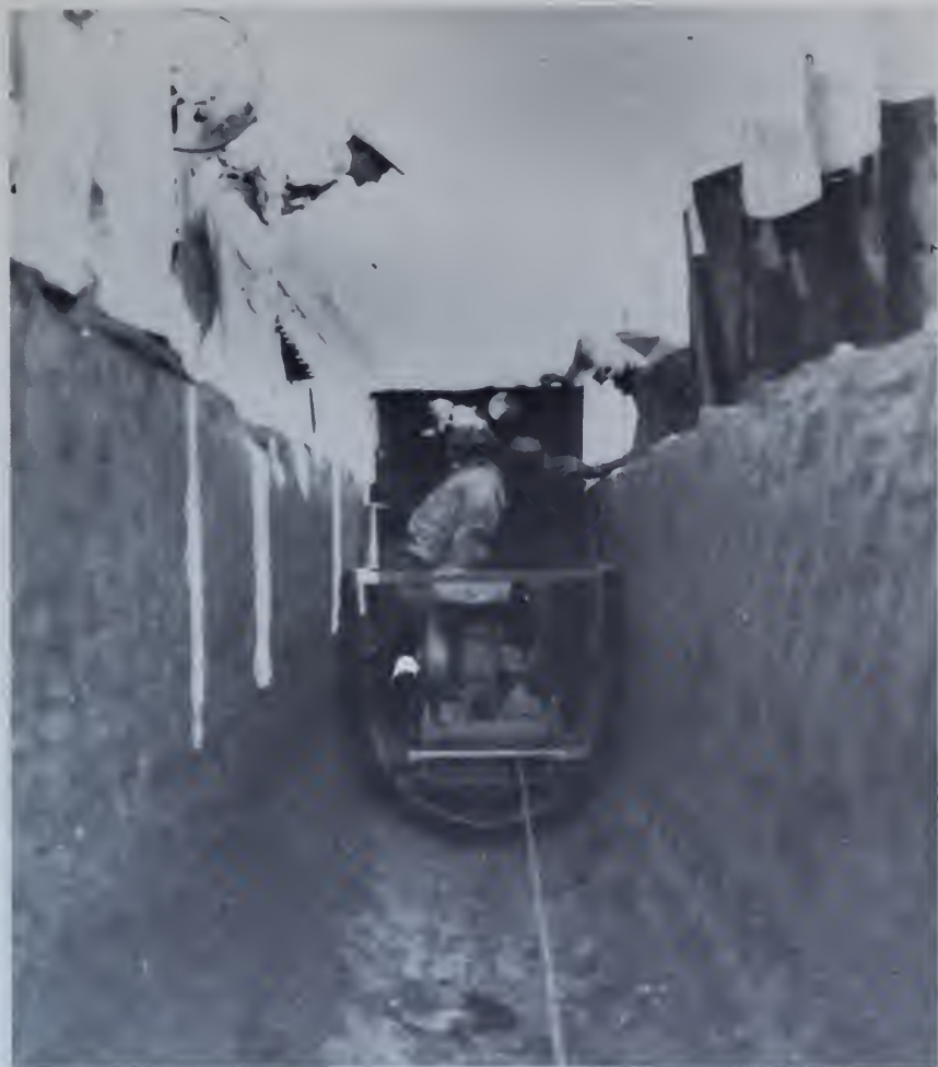
Figure 170.—Placement of cast-in-place concrete pipe. Concrete, transported by truck mixer, is being dumped from the left side into the placing machine. PX-D-34074.
